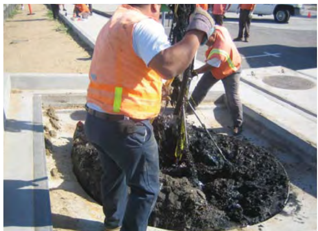
Exhibit 2.4 Maintenance and cleaning
