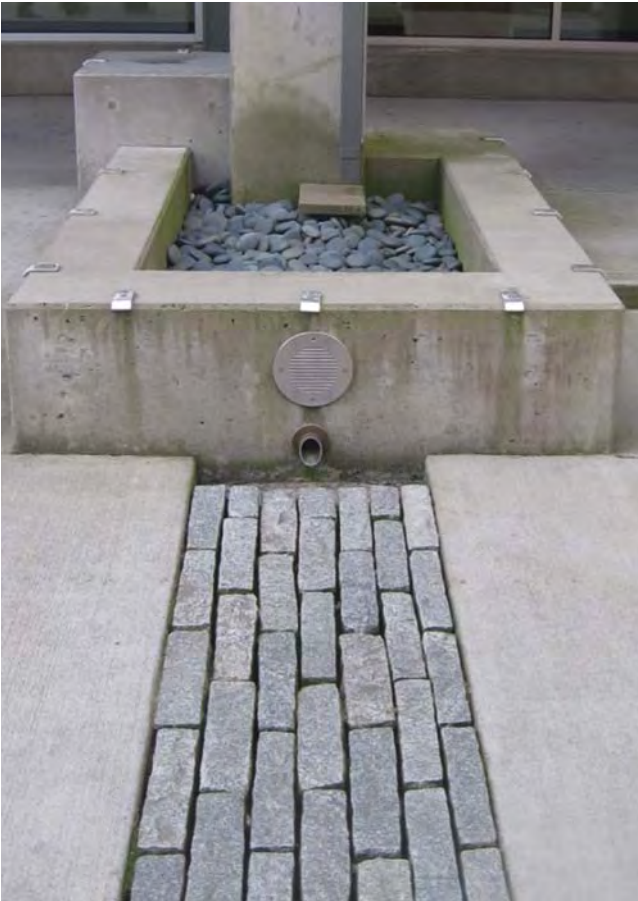
Exhibit 2.18 A rainwater downpipe draining to an open landscaped surface water box
