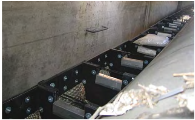
Exhibit 2.27 A line of ultra-urban filter inserts in an LA catchpit
