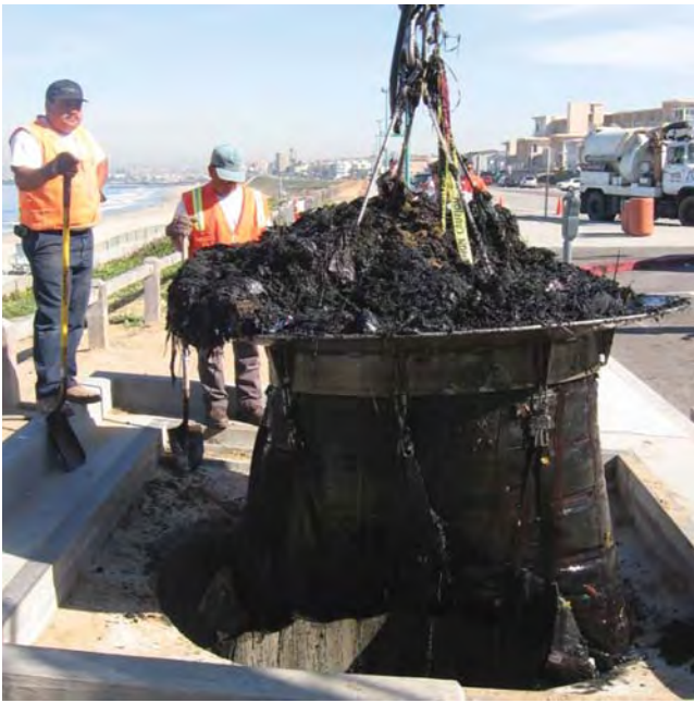
Exhibit 2.28 Essential cyclic maintenance on a CDS Technologies installation; removing LA's trash
