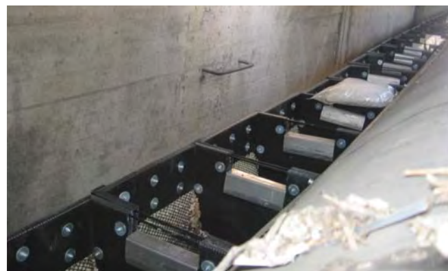
Exhibit C.20 A line of ultra-urban filter inserts in an LA catchpit
