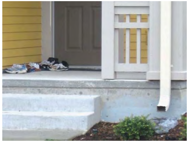
Exhibit 2.19 Downpipe disconnection is simple, cost effective and it works
