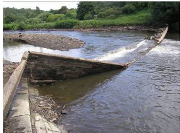
River Irwell near Little Lever, weir collapses following record rainfall event
